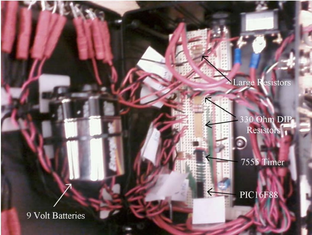
Figure 10: Inside View of Circuit Box
